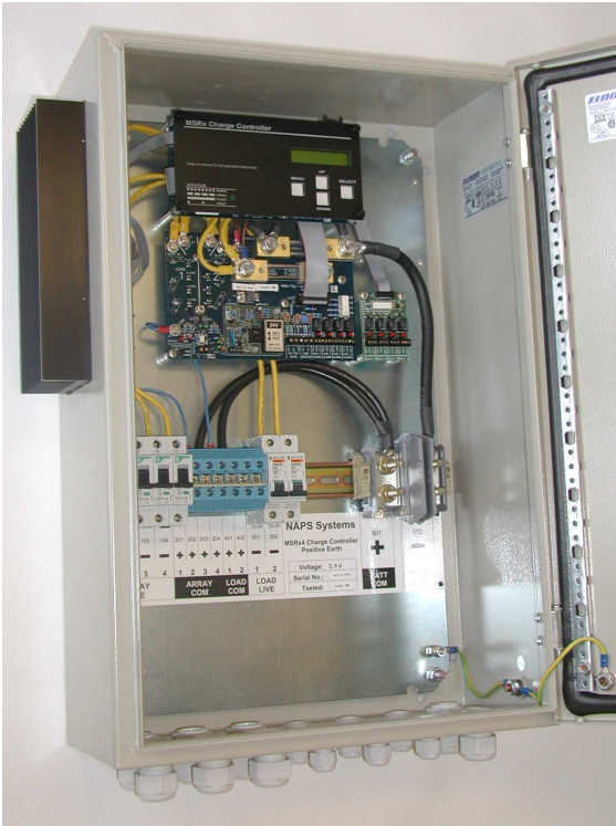
The MSRx4 in Painted Steel Enclosure
